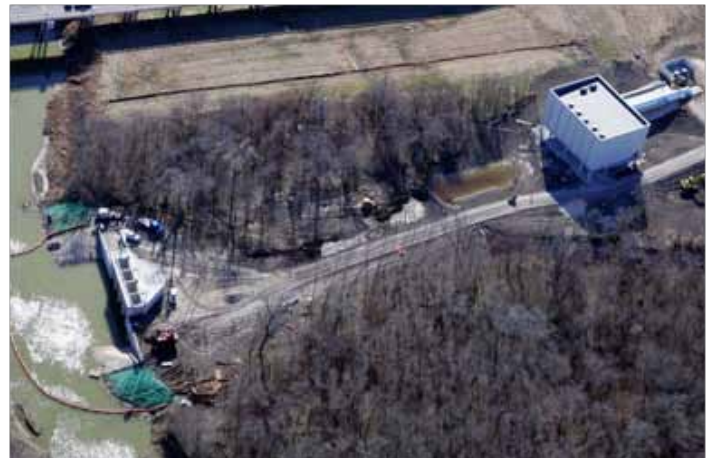
East Fork Diversion Pump Station
