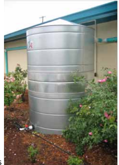
A large storage tank to store rainwater from the roof
